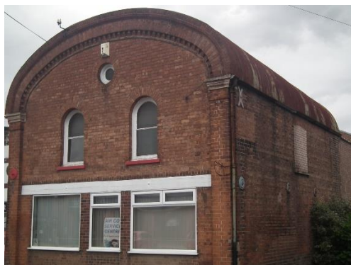
It's not listed, but it is curious, especially as the tin roof looks original
